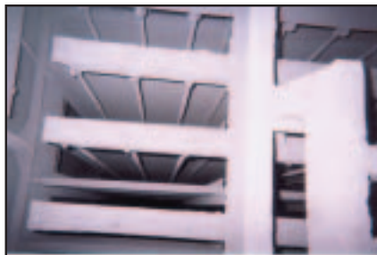
Figure 4 Ash buildup on collecting plates and discharge electrodes.
