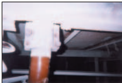
Figure 5 Loose and missing bolts on an emitting system vibrator shaft identified during a clean inspection.
