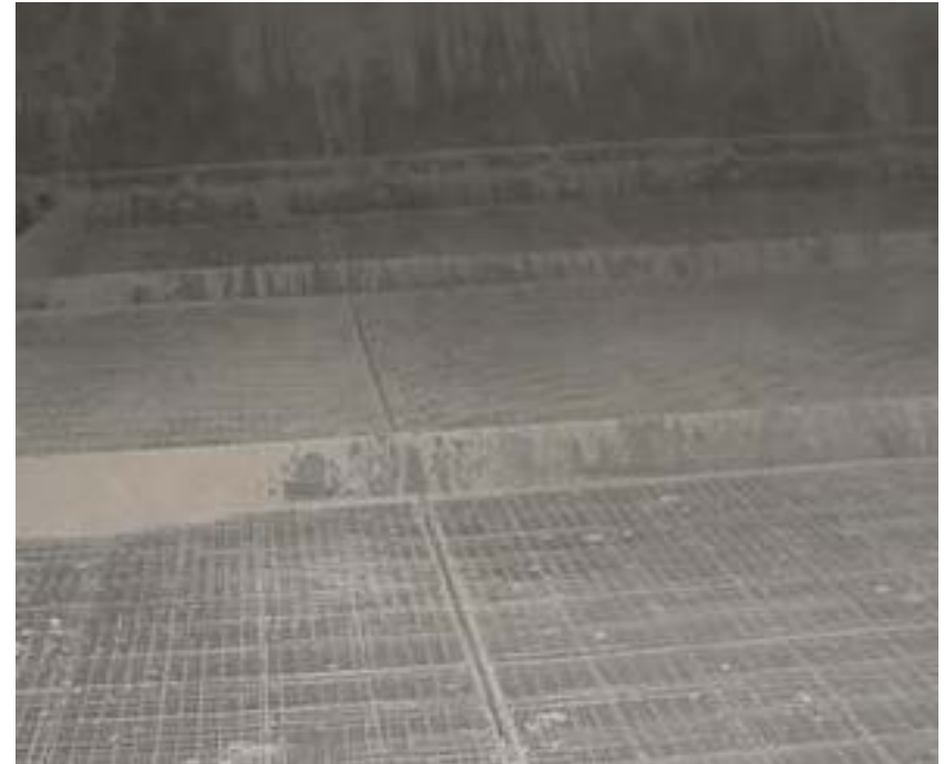
High Dust Reactor
