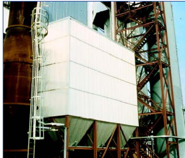
Coal-fired Industrial Boiler 110,000 ACFM
