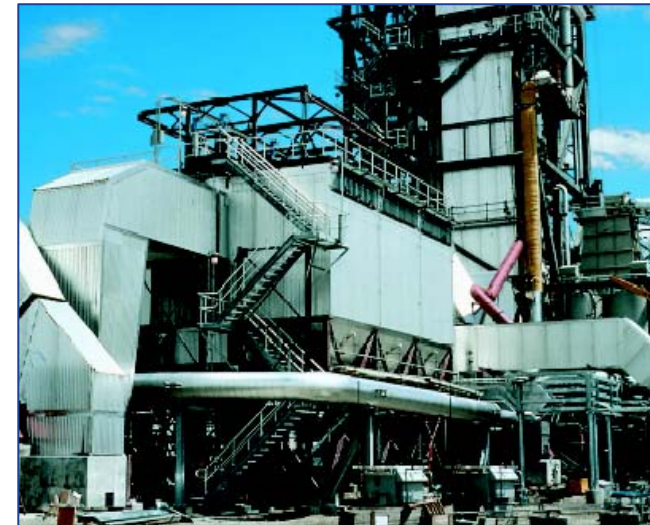
Utility Boiler 500,000+ ACFM
