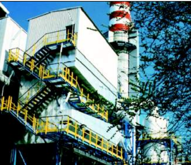
Municipal Solid Waste Incineration 16 MW – 65,000 ACFM
