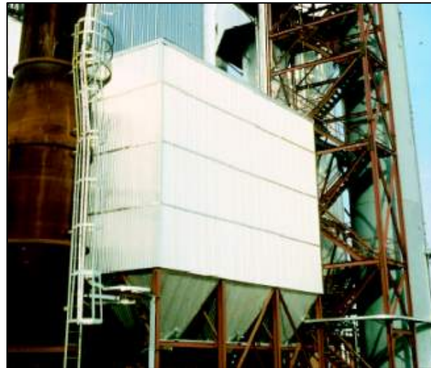
Coal-fired Industrial Boiler 110,000 ACFM
