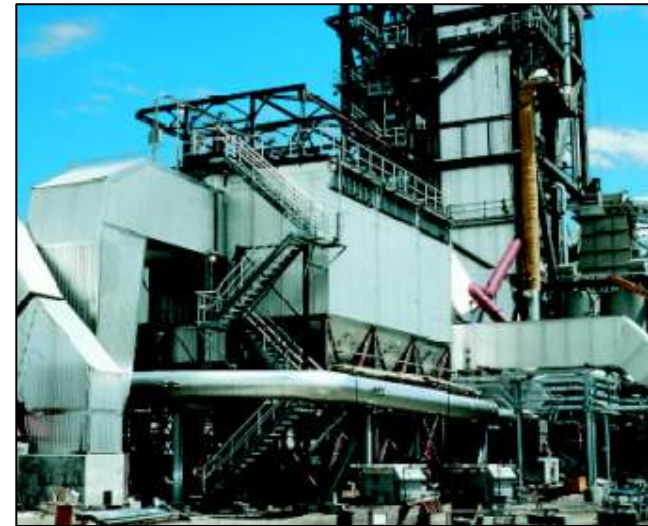
Utility Boiler 500,000+ ACFM
